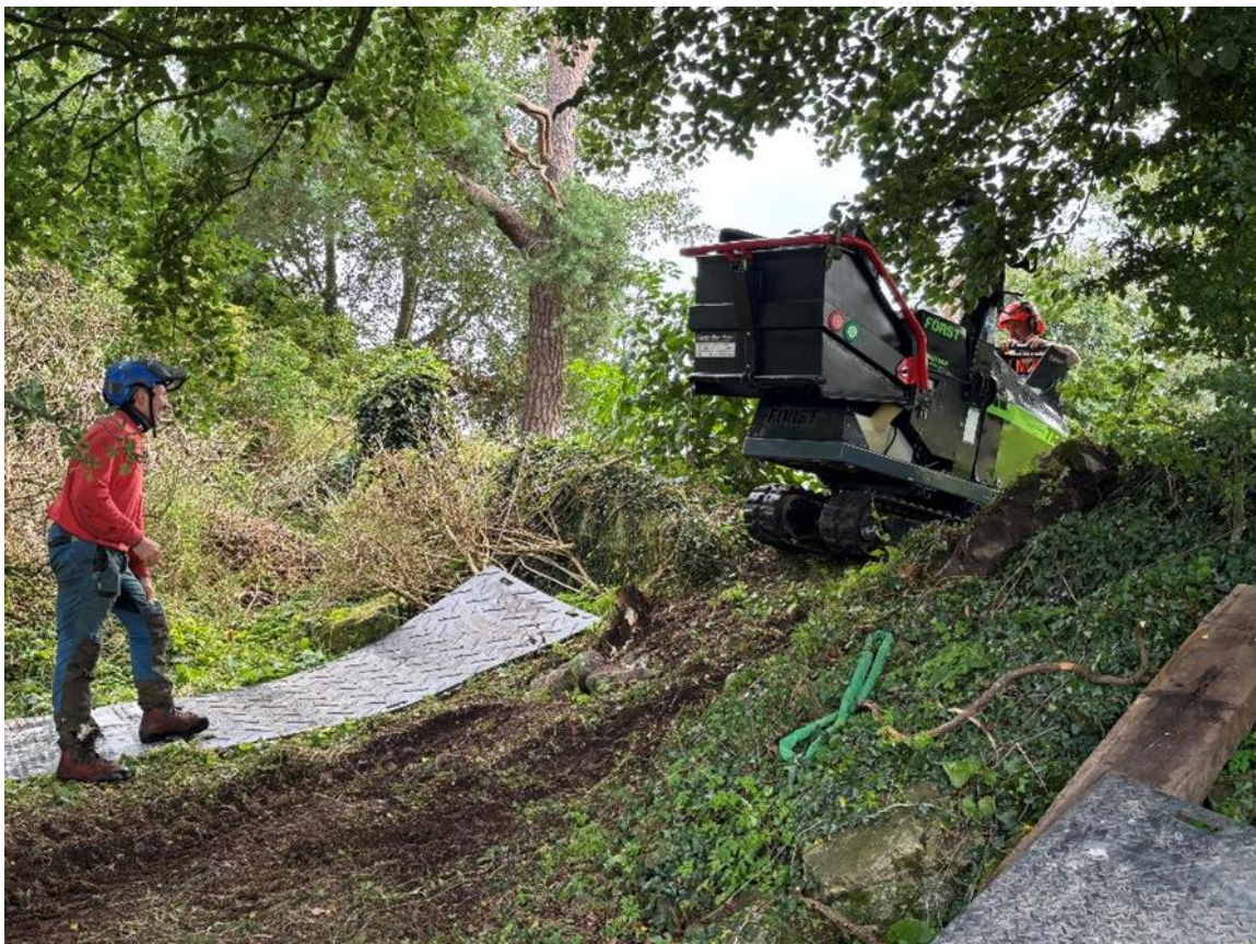
Figure 5.14: Plastic matting being placed down in advance of crossing the enclosure bank.
