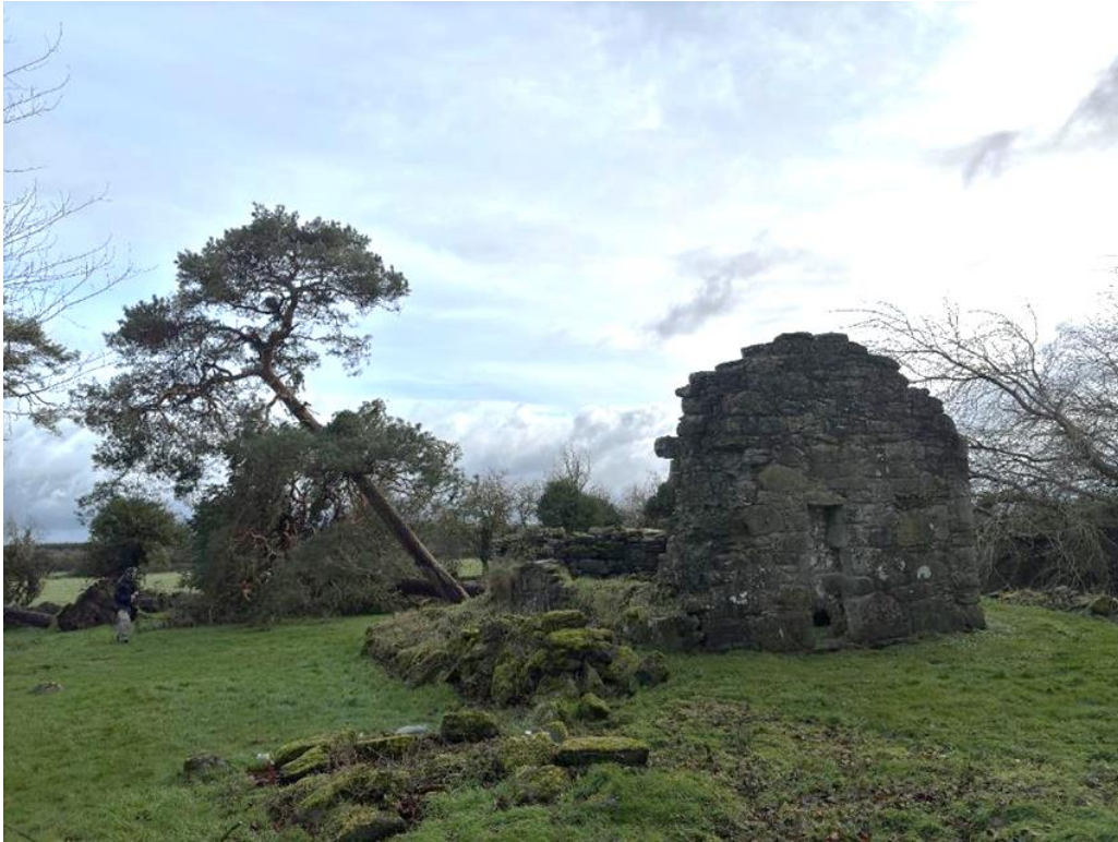
Figure 5.1: The site, shortly after Storm Eowyn, as reported to the NMS and NMI on 28 January.
